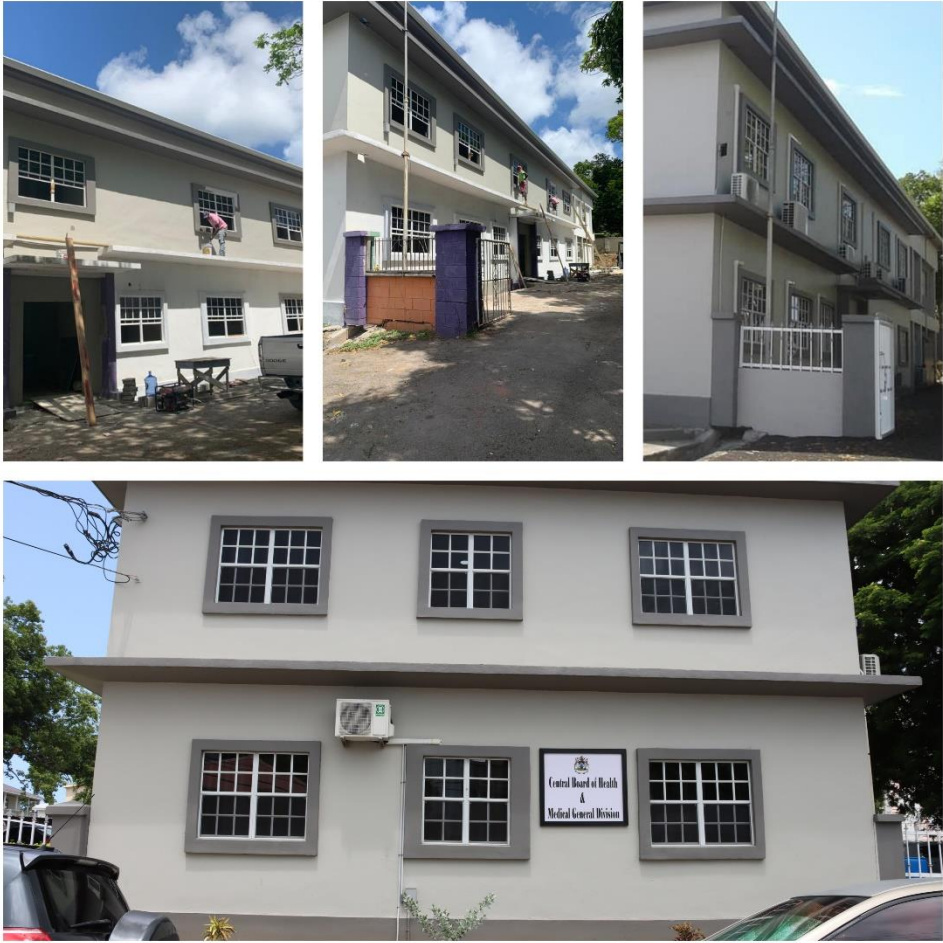
Picture 16: Collage of Completely Renovated Premises for the Central Board of Health
